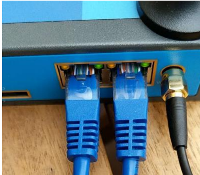
Figure 2.4 Connect Ethernet cables
